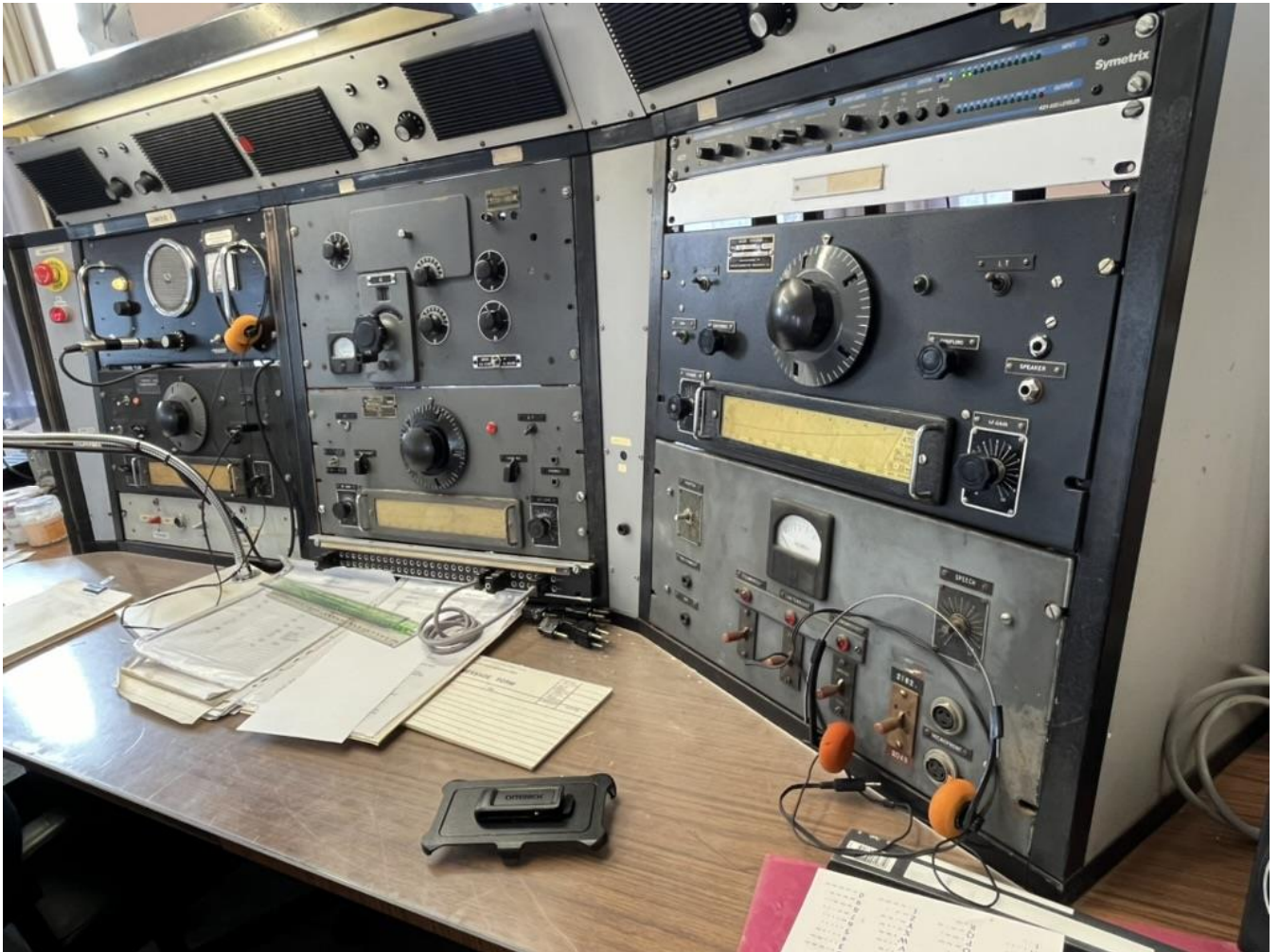
Newly-installed 941 Receiver (Right hand panel) at Musick Point.
