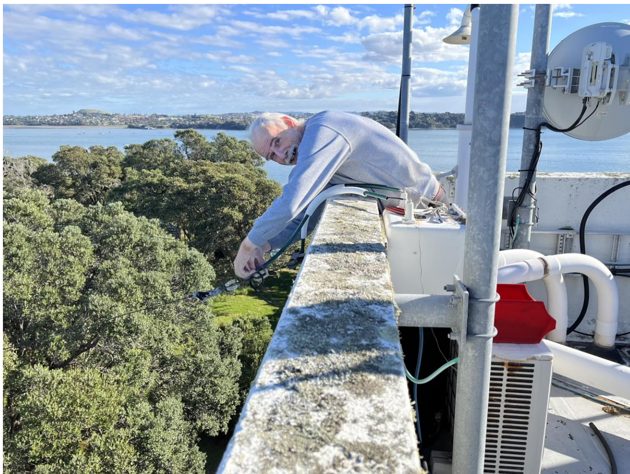
Ah- the sweet smile of success! Harry ZL1BK completing the rejoining of the Vee Beam on the ZLD tower roof, on a recent beautiful autumn day.
