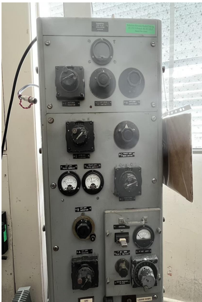
RCA 80 meter Vintage Transmitter at Musick Point
