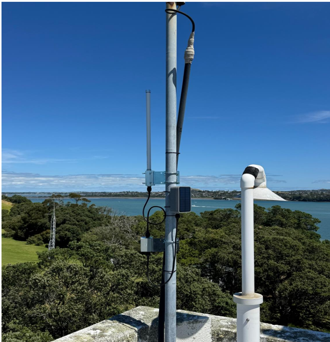
The new "Meshtastic" Node installation at Musick Point Radio Station. (details below)
