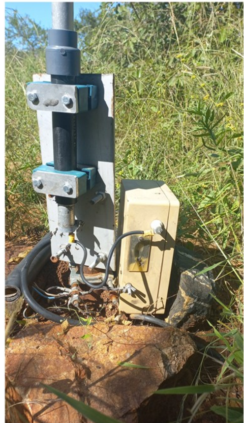
Fig. 2 – Antenna base showing clamps, mounting plate and weatherproof box containing the matching circuits and relays
