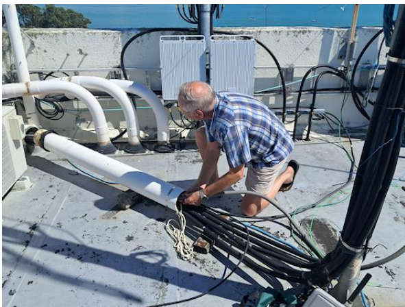
Who said this duct is large enough for more cables?
