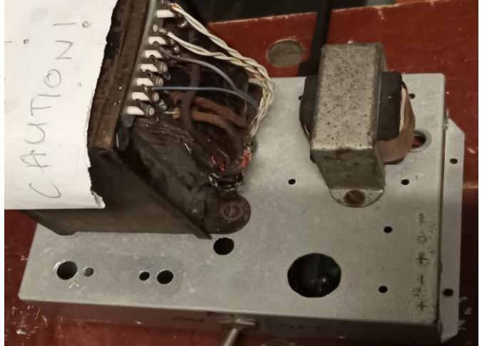
Power supply- before...(Shock! Horror)! Exposed AC mains terminals, not an isolated finding at MP)
